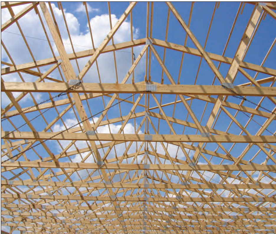
Figure 35. Typical Post-frame roof framing showing engineered metal plate connected wood trusses, roof purlins affixed atop trusses on edge and lower chord stiffeners.
